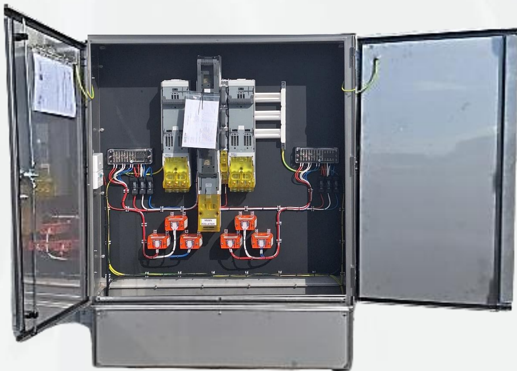
Aitutaki Power Supply Cook Islands.
