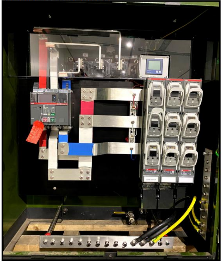
1600 AMP ABB ACB WITH 3 WAY LV RACK
